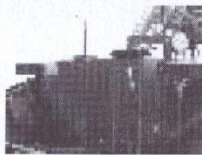
Hydraulic Oil Tank
