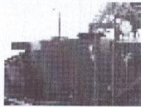
Hydraulic Oil Tank
